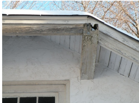
16. Rotted roof purlin ends
