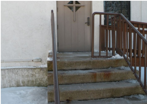
9. Displaced railings at side entry
