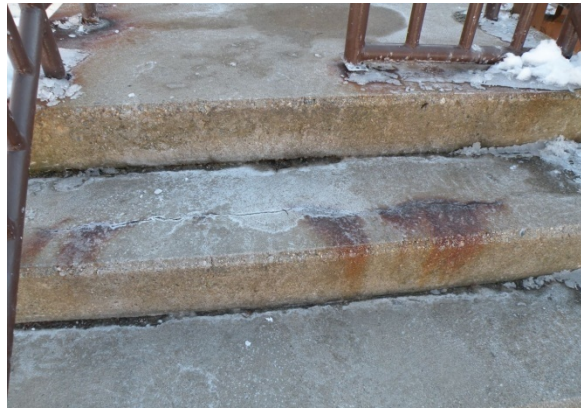
10. Cracked stair treads at side entry
